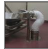
LEV (Local Exhaust Ventilation)
